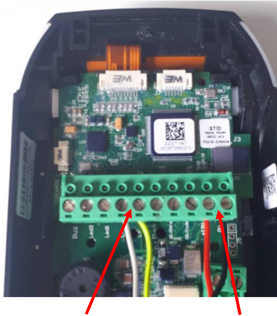
Reader RS485 bus 12VDC power supply bridged with the ones of the access control module
